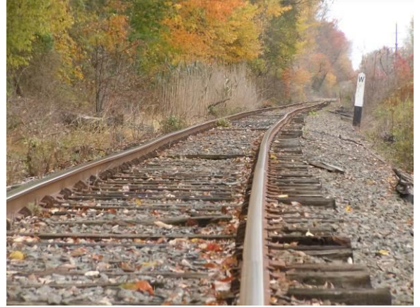
Existing warp, surface irregularity, and line deviation at South spiral.
